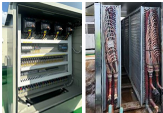
<Implementation of Energy Efficiency Improvement Equipment>
