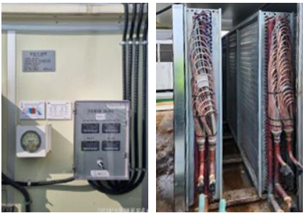
<AHU Heat Pipe Dehumidification System>
